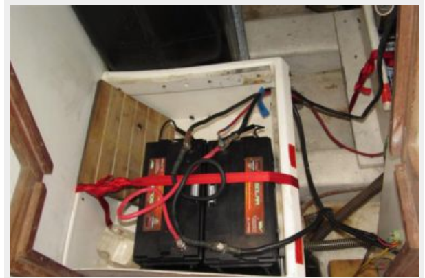
Batteries in Storage under stairs
