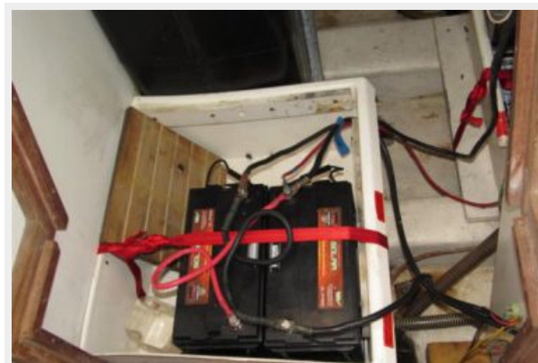
Batteries in Storage under stairs
