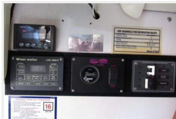
Gauges and monitors at nav station
