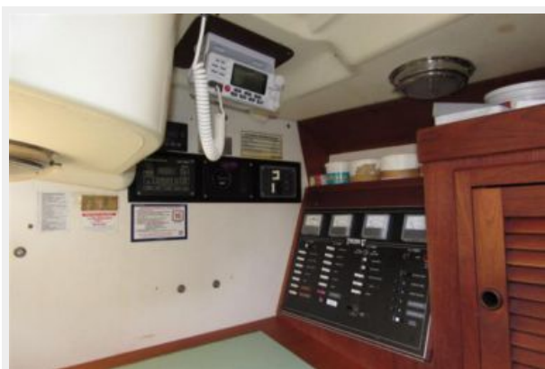
Electrical panel and electronics at nav station
