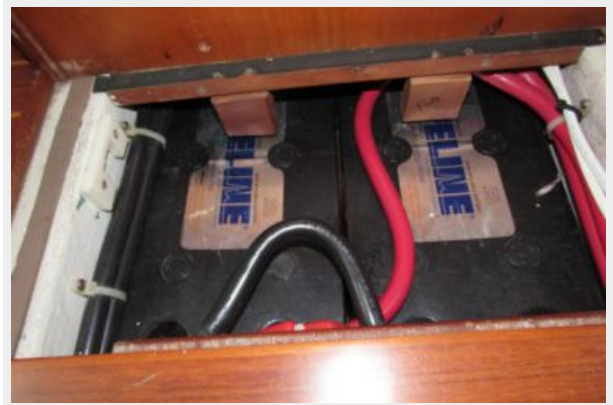
Battery storage under floorboards
