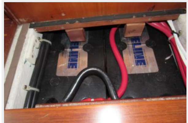
Battery storage under floorboards
