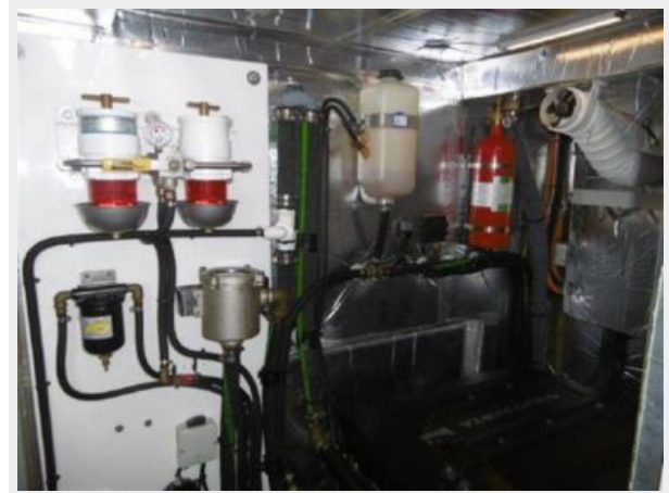
Good access in the engine room
