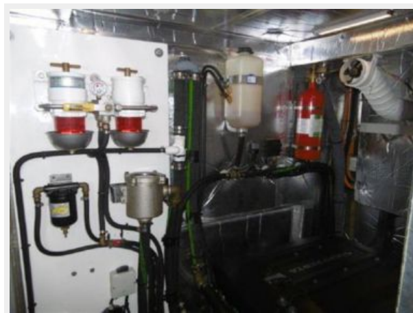
Good access in the engine room
