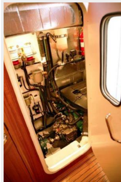
Engine room access with door
