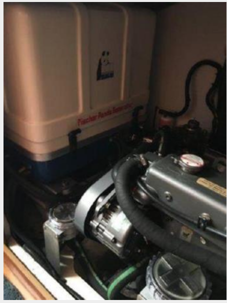
Clean, orderly engine room
