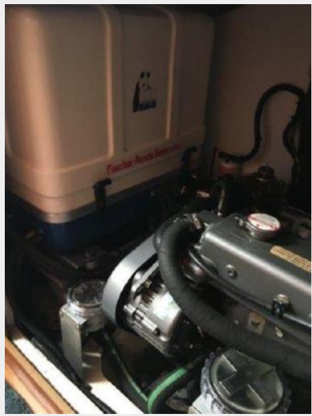
Clean, orderly engine room
