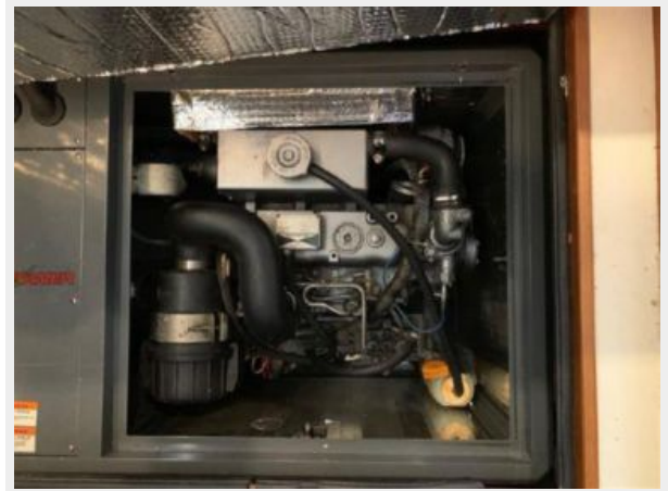
MASPOWER 8KW GENSET
