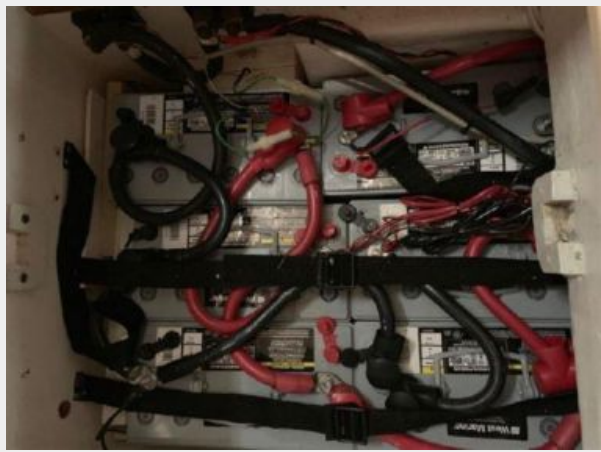
HOUSE BATTERY BANK
