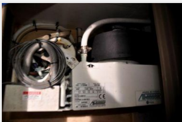
One of three AC units
