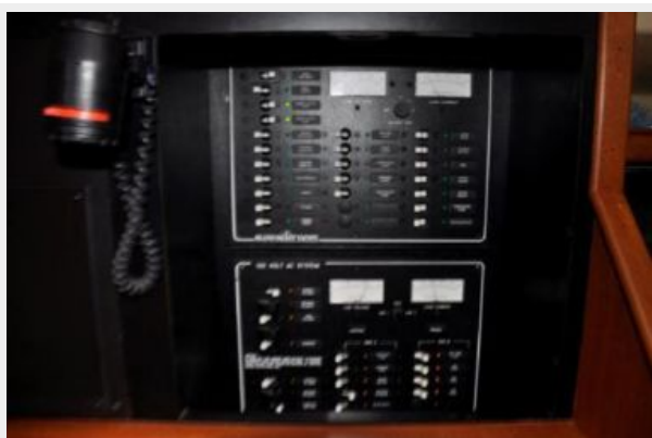
AC and DC control panels
