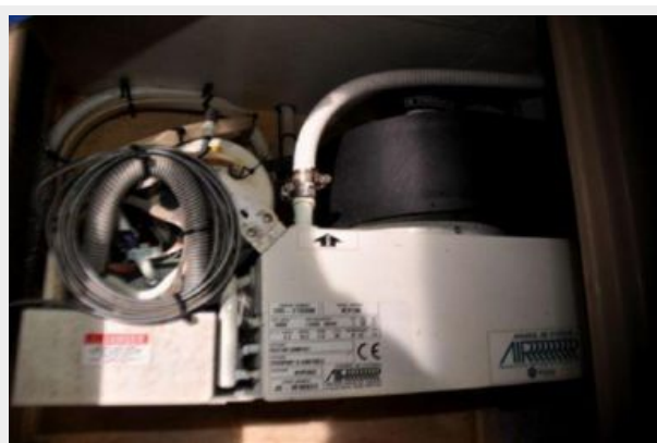
One of three AC units
