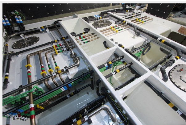
Piping Runs in Bilge
