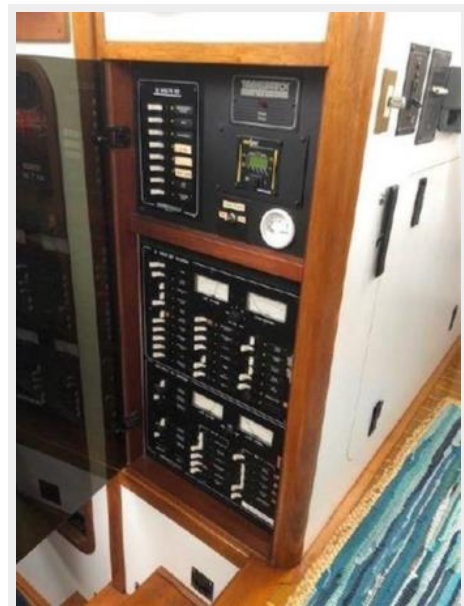
Electric Panels at Companionway
