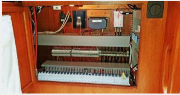
Breaker Panel Access
