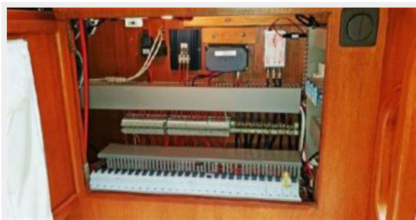
Breaker Panel Access
