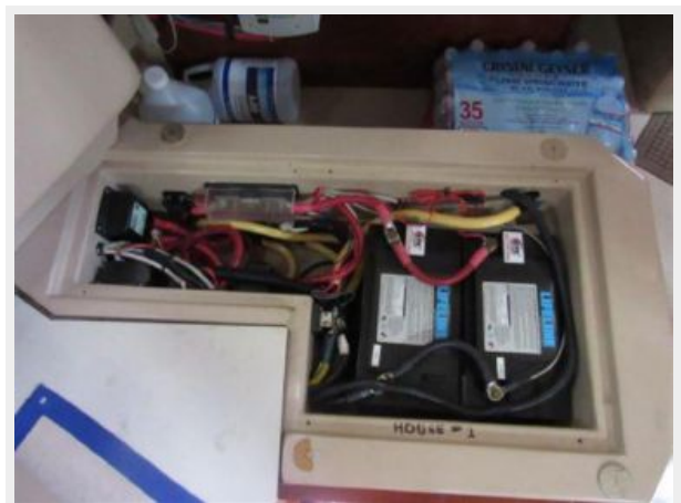
Battery storage under nav seat
