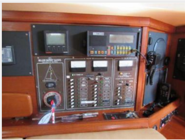
Elec Panel at Nav Station
