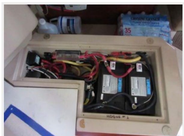
Battery storage under nav seat
