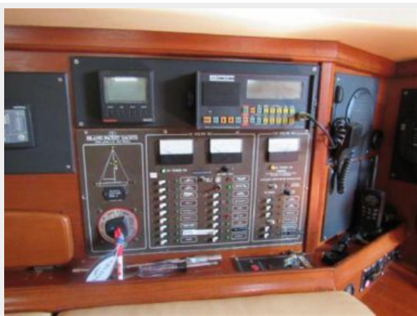
Elec Panel at Nav Station
