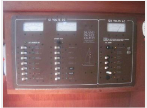
12 V + 110V Electrical Panel
