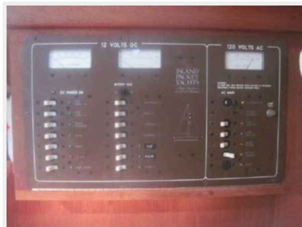
12 V + 110V Electrical Panel
