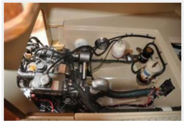
Spotless Engine Room
