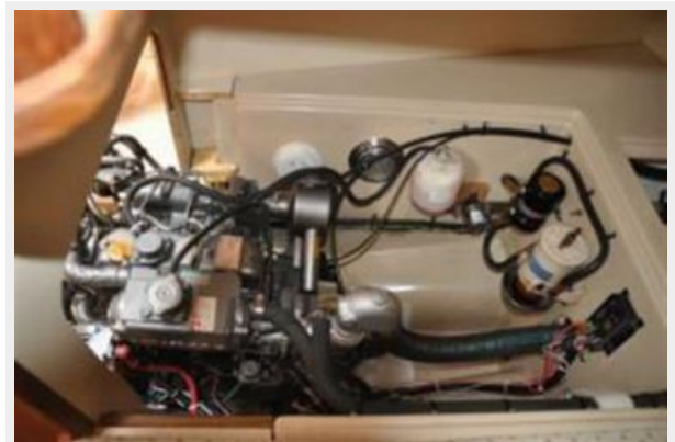
Spotless Engine Room
