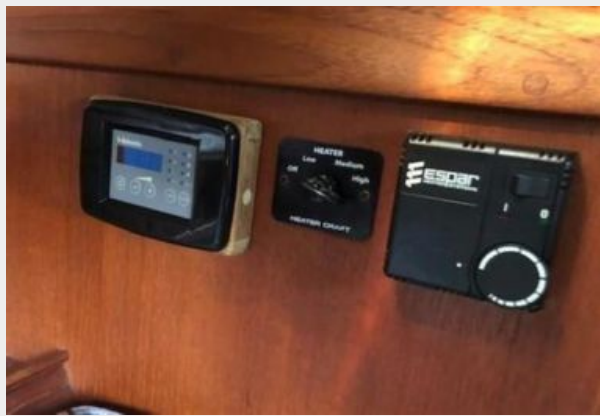
Diesel Heater & Heat Pump Controls
