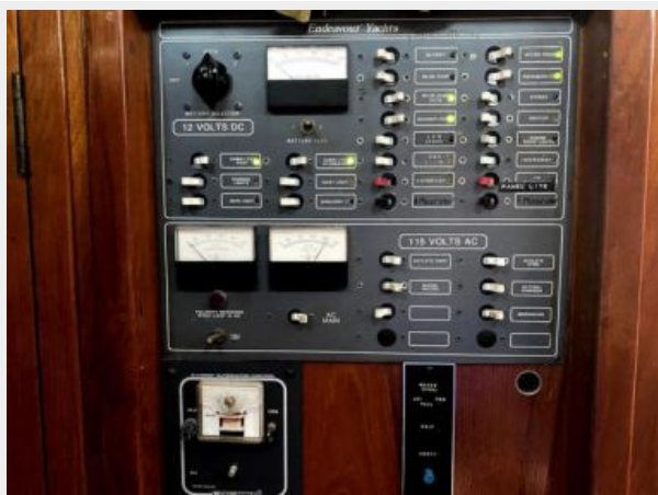
AC/DC control panel
