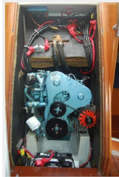
Perkins Engine compartment
