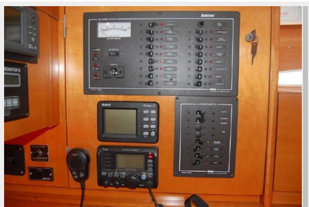
DC / AC Electrical panels, Auto Pilot, VHF radio
