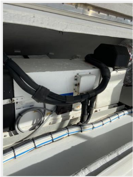
AC in bridge
