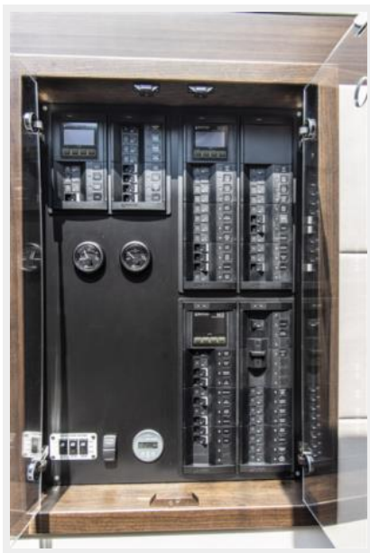
Companionway electric panel
