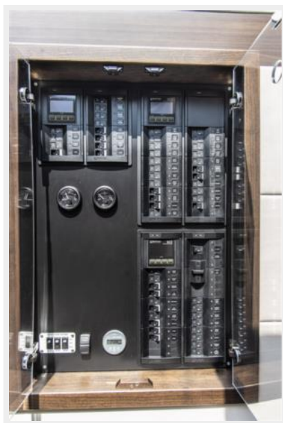
Companionway electric panel
