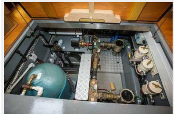
Easy Access to Plumbing
