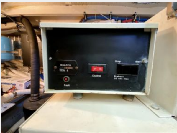
Generator controls and hour meter
