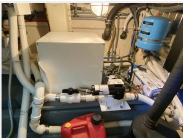
2017 New water heater
