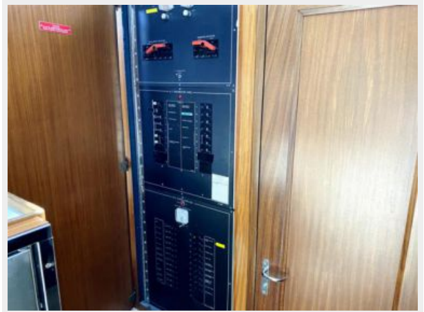
AC/DC electric panel
