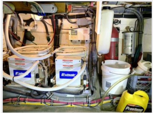
starboard forward engine bay with 2010 AC units
