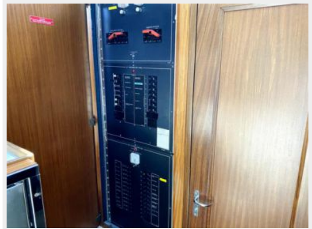
AC/DC electric panel
