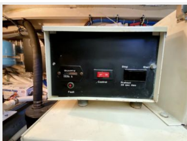
Generator controls and hour meter
