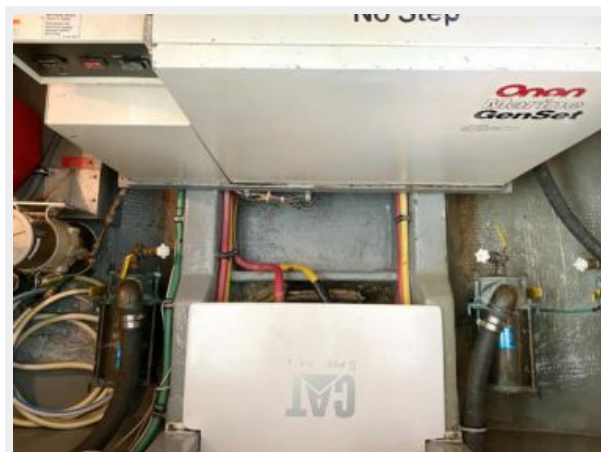
spotless engine room and bilge
