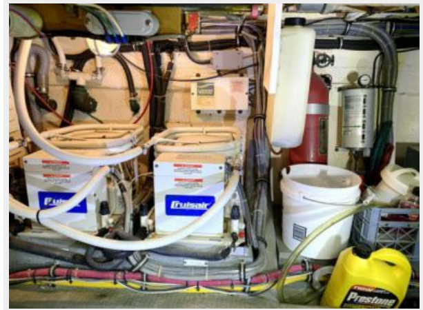
starboard forward engine bay with 2010 AC units
