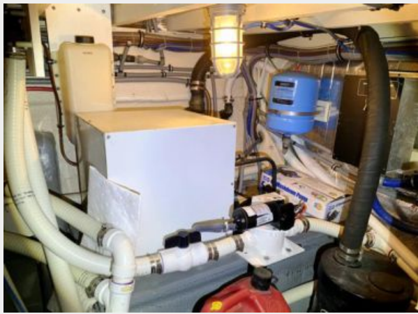
port forward engine bay with 2017 water heater
