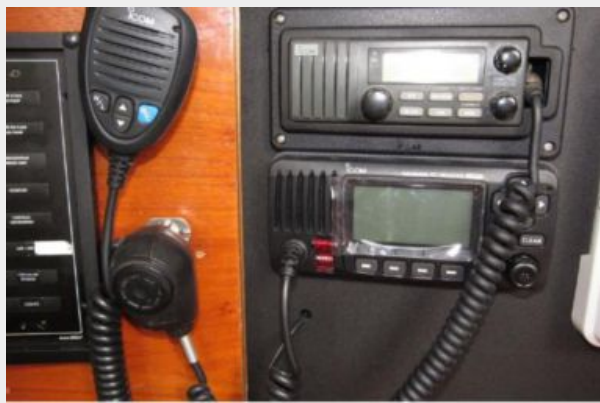
Instruments at nav station
