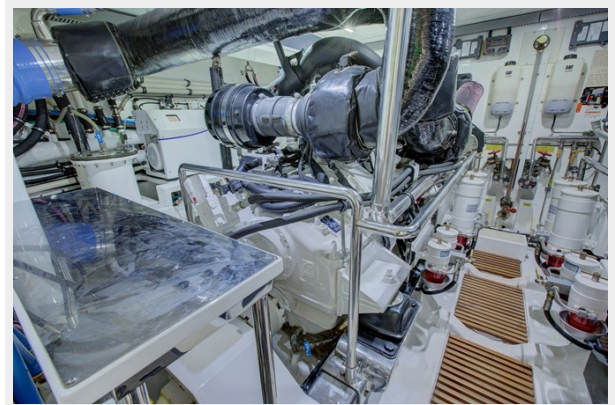
Engine Room Looking Port
