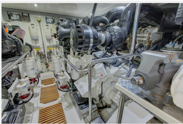
Engine Room Looking Starboard
