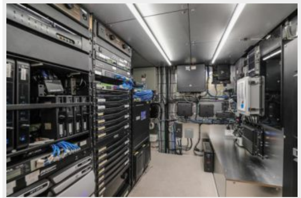
A/V and Electronics Room
