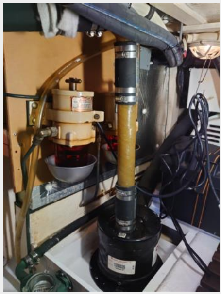
Generator: dual Racor filters, exhaust, muffler
