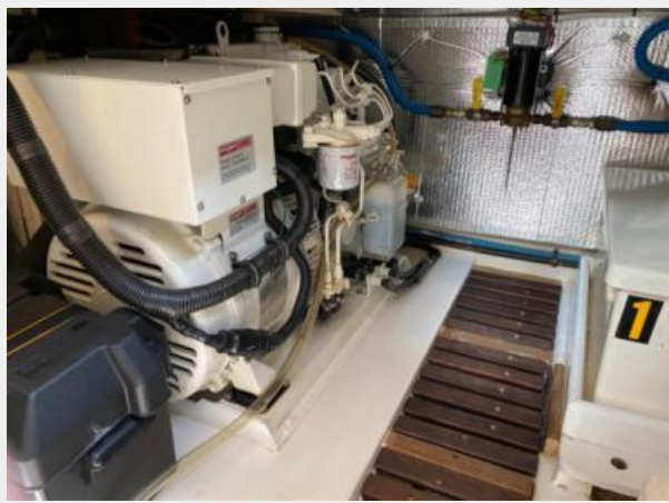
Northern Lights 8kW generator, teak grating in engine room, fiberglass battery box
