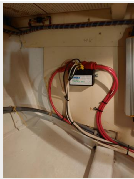
Imtra Windlass Control Box mounted in Engine Room
