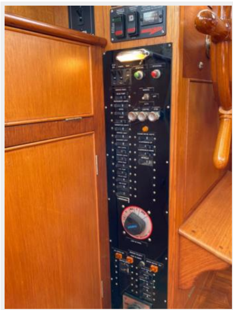
AC/DC Control Panel at Lower Helm
