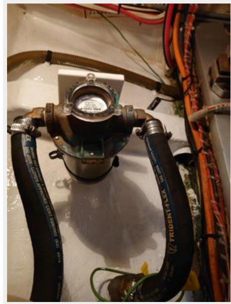
Engine: Groco raw water strainer
