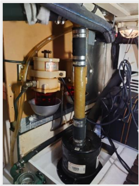
Generator: dual Racor filters, exhaust, muffler
