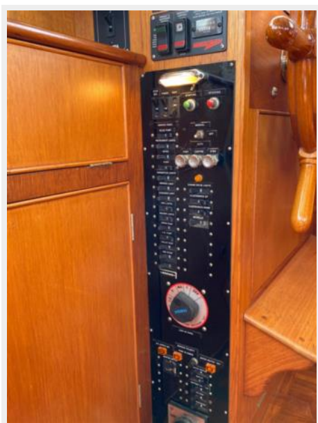
AC/DC Control Panel at Lower Helm
