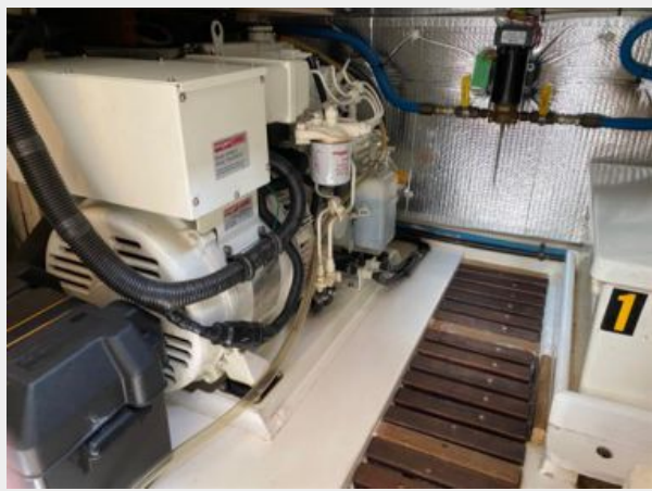
Northern Lights 8kW generator, teak grating in engine room, fiberglass battery box
