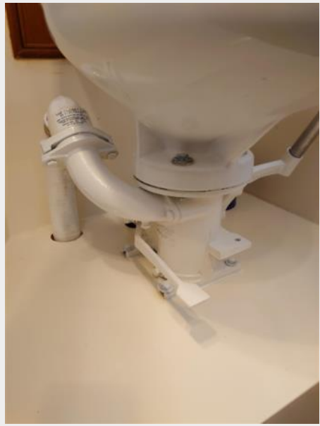
Marine toilet: no leaks here!
