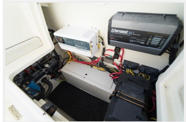
2016 32 World Cat Engine Room
