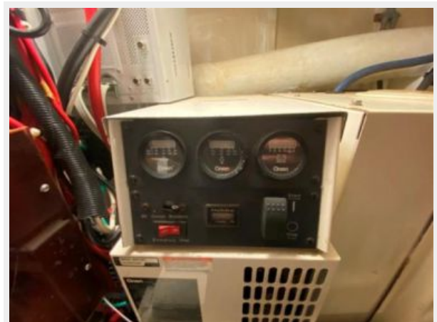
331 Generator Control Panel
