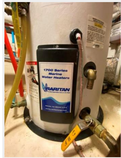
321 Hot Water Htr
