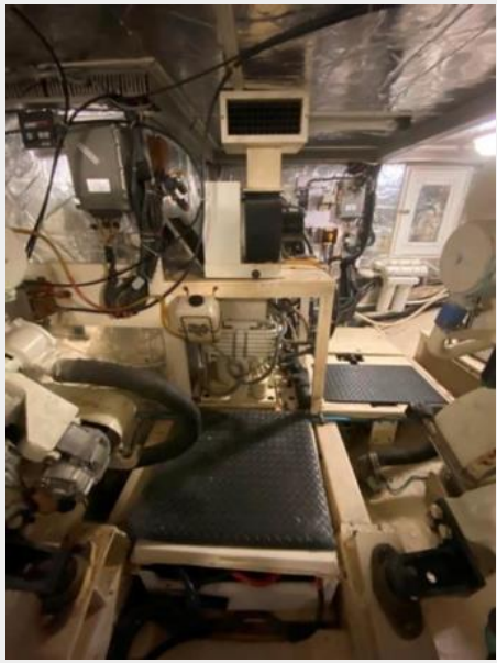
326 Engine Room Fwd
