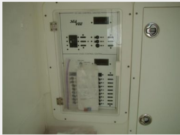
25. Breaker Box located in Head
