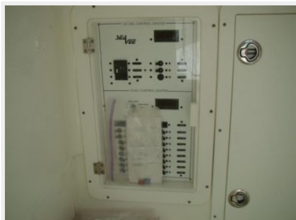
25. Breaker Box located in Head
