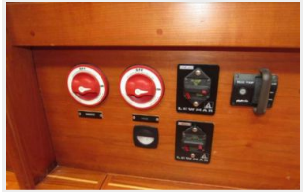
Battery and breaker switches
