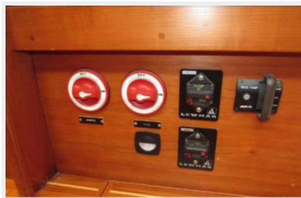
Battery and breaker switches
