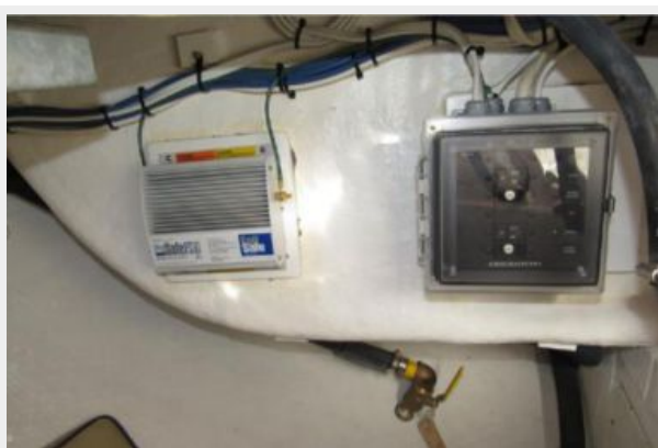
Galvanic isolater and ELCI controls
