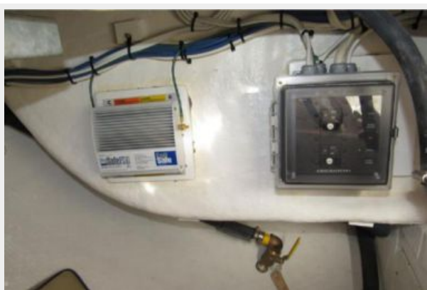
Galvanic isolater and ELCI controls
