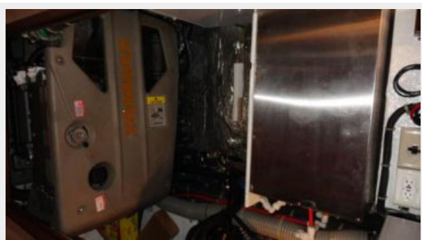
Engine Room Fwd.
