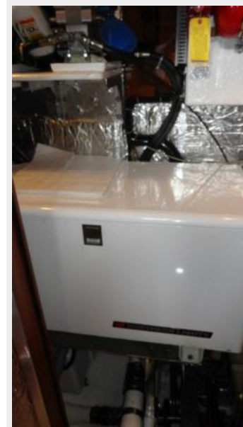
Engine Room Aft
