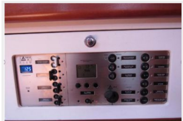
DC electrical panel
