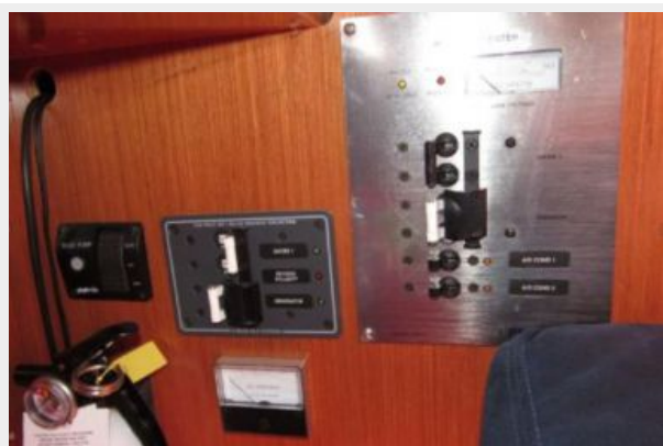
AC electrical panels
