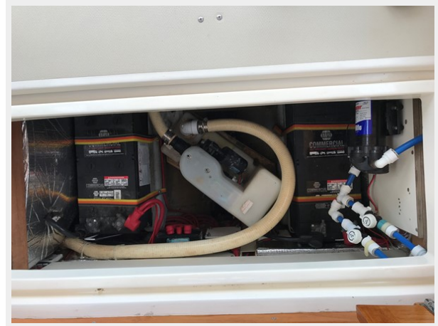
Pump and Battery Room
