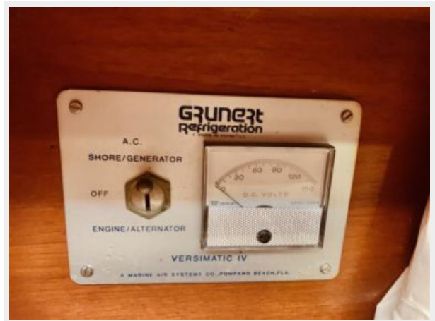
44.1 Little Red 1984 Grand Banks 49 MY refrigerator power control 1
