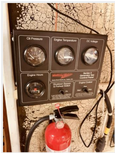
94 Little Red 1984 Grand Banks 49 MY generator controls
